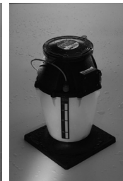
Liquid Chlorine Container
